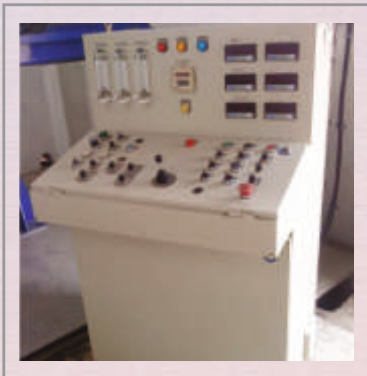
Main Control panel
